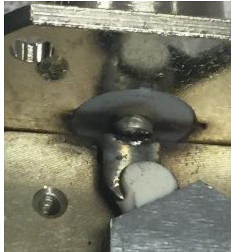
Broken solder joint at output connector caused arcing
